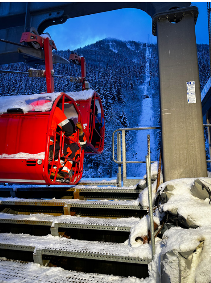
Maintaining and replacing planetary gearboxes on a ski lift in Europe comes with a unique set of challenges.
