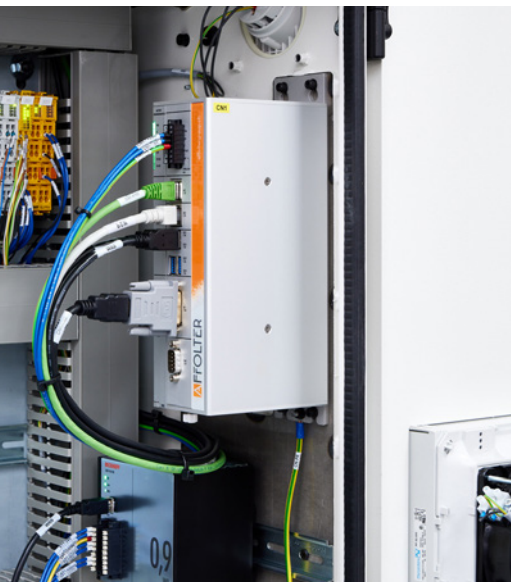
Control for the lathes: The C6920 control cabinet Industrial PC (right), which runs the TwinCAT CNC for up to twelve servo axes and spindles, and the associated EtherCAT Terminal system (left).
