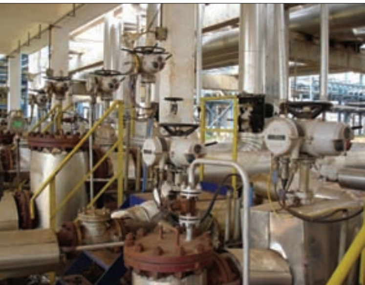
Rotork IQPro valve actuators were installed in a processing area of the Qinzhou Refinery.
