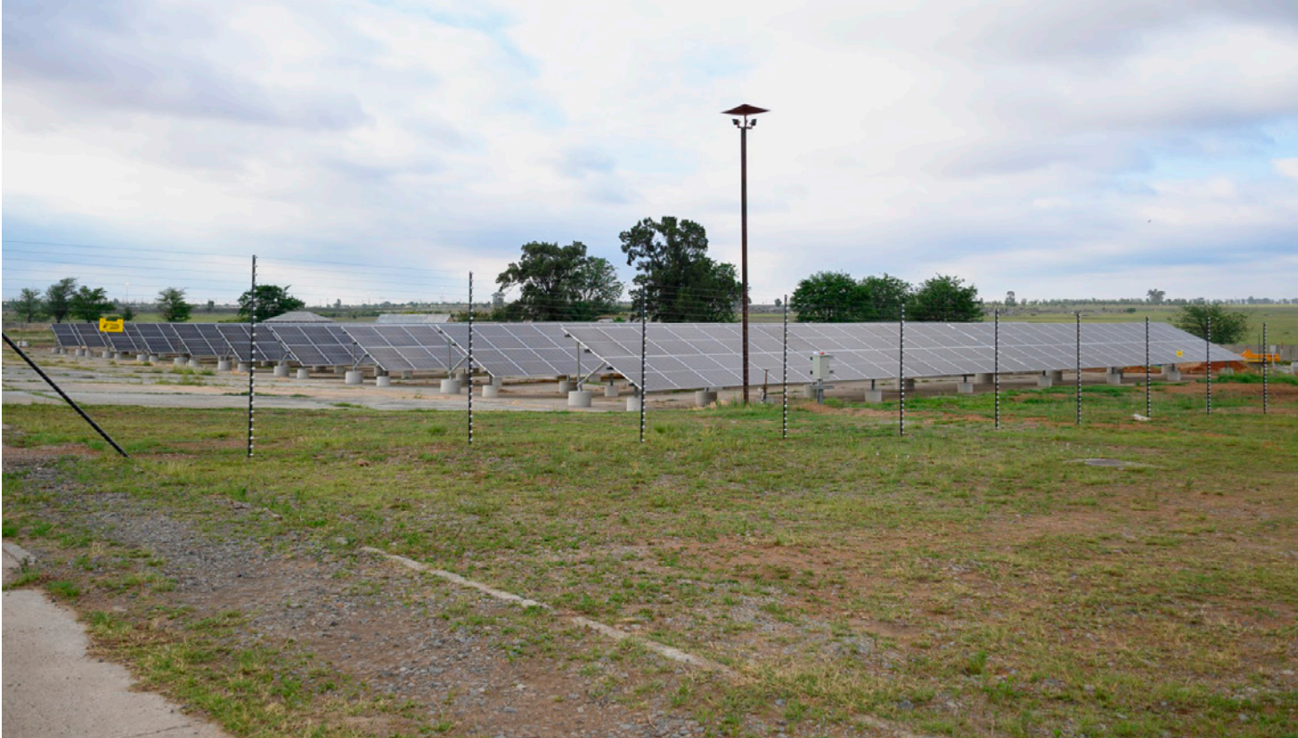
On-site at Vesconite Bearings, where the company is installing a comprehensive solar energy solution.
