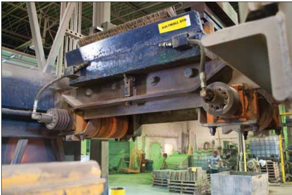
A single production line at Reading Rock means any problems could bring the entire production line to a halt (all photos courtesy of Force Control).
