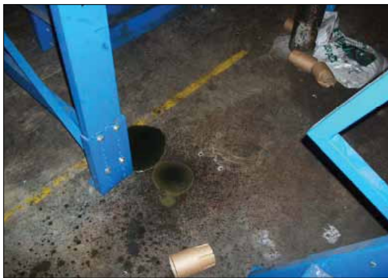
Figure 8—Example of seal failure.
