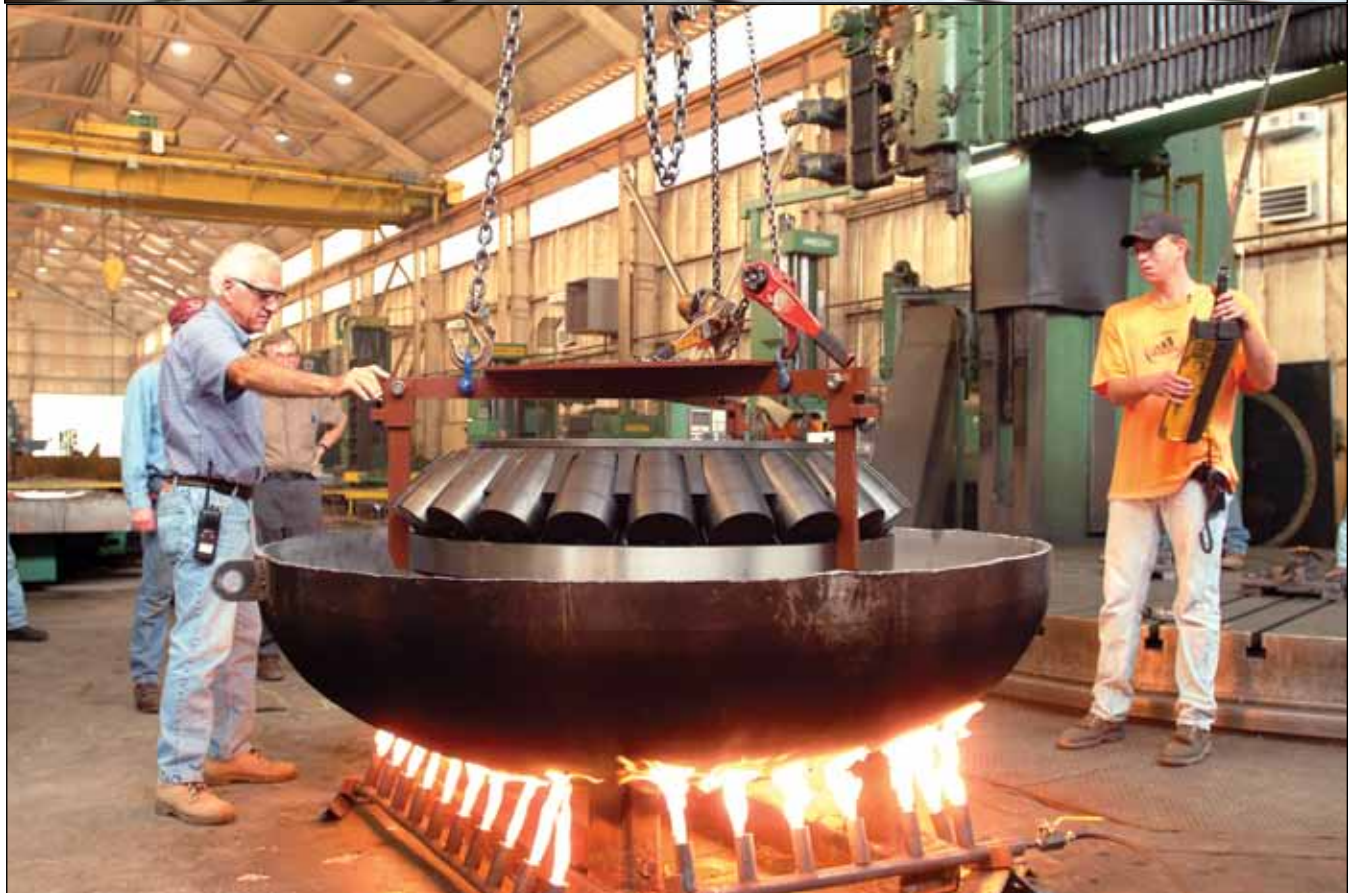
The final mounting and horizontal preheat of a large bearing for a New York bridge application (courtesy of SKF).
