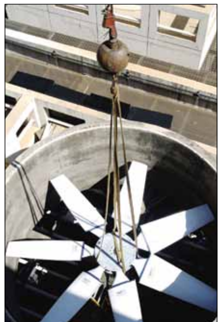
Rod Applegate, owner and president of Tower Engineering, Inc., says the Baldor engineers were smart enough to create a low profile motor design that fits in the same space and mounting footprint as the gearbox.
