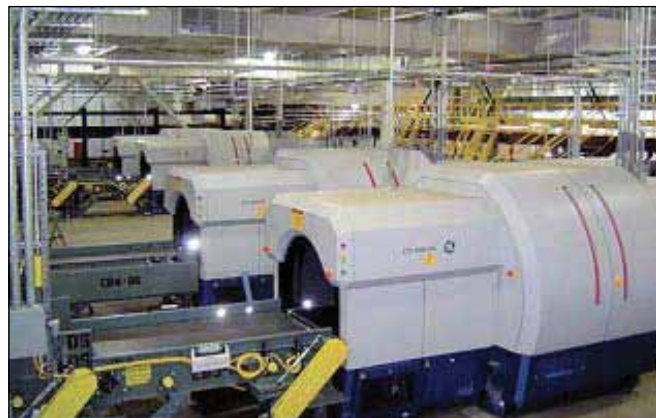
Figure 2—Inline EDS and queue conveyor (Ref. 10).
