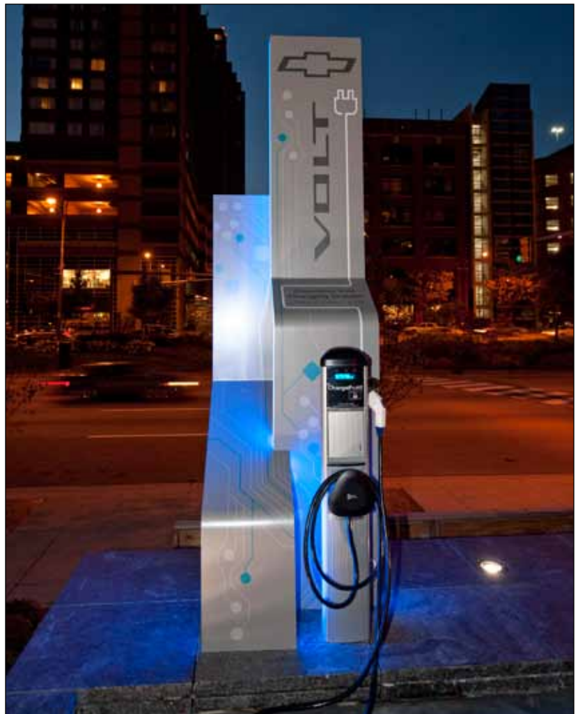
The cost, availability and accessibility of charging stations like the one pictured above will dictate the acceptance and popularity of electric vehicles. GM recently announced that “more than 5,300 home and workplace” stations will be installed throughout Michigan in the coming year.
